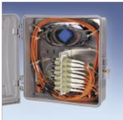
OPN-1224 shown with customer provided cabling, adapter plates and adapters.
